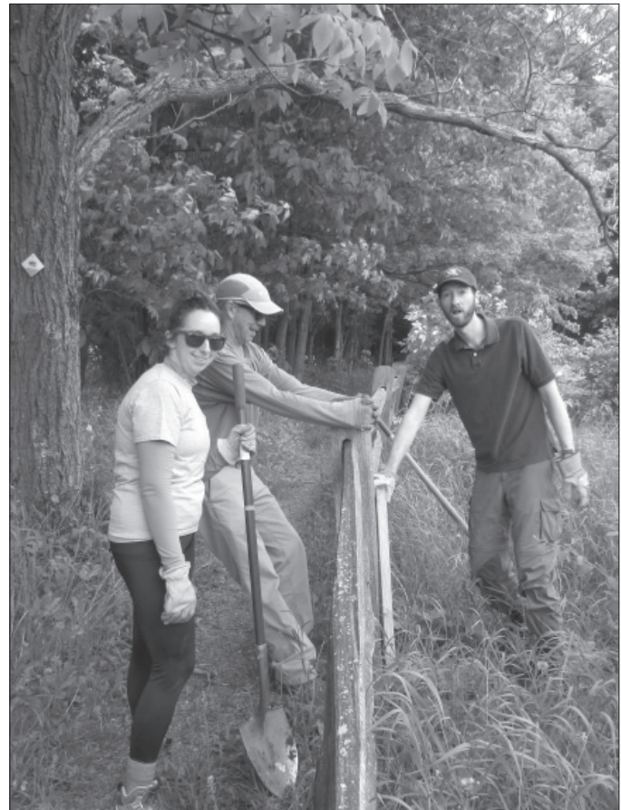
Repairing the fence line at the Landon Community Trail with Jeff from Lake Champlain Land Trust
