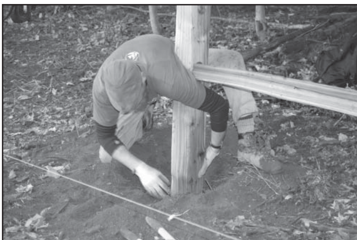
Josh Ryan of Timber & Stone LLC places a cedar fence post solidly in the rocky soil.
